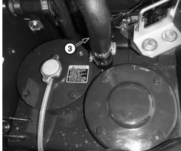
Hydraulic Oil Return Line
