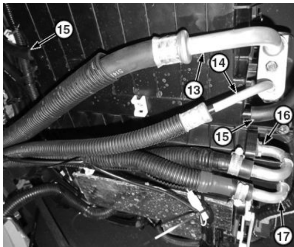
Heater and Air Conditioner Lines
